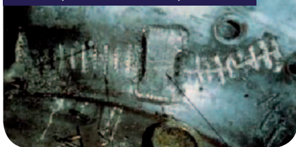
Figure 4: front wall of cement mill after carrying out repair with metallock method (source: Munich Re)
